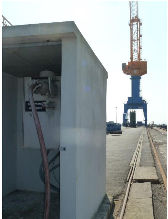
3PX6 24KV BREST HARBOUR FRANCE
